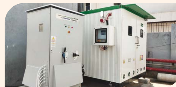
Flipkart – 1.88 MWp Rooftop Solar + 770 kWh BESS in Maharashtra
