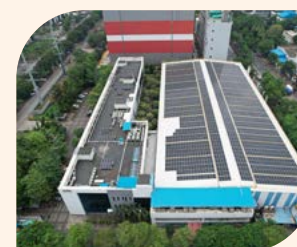
Parker Hannifin 1.16 MWp Rooftop Solar System in Mumbai
