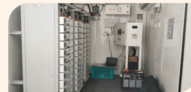
D-Mart – 450 kWp Rooftop Solar + 234 kWh BESS in Bengaluru
