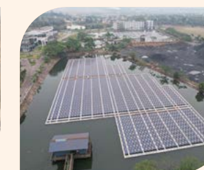
Shyam Metalics 1.2 MWp Floating Solar System in Sambalpur
