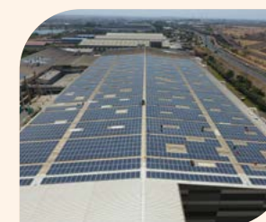
Ferrero India 2.44 MWp Rooftop Solar System in Pune
