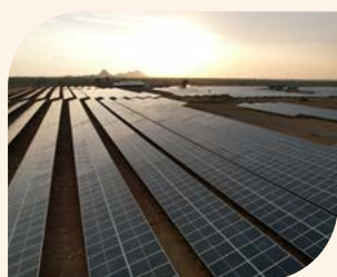
Dhule, Maharashtra (MH-2) -150 MWp Solar Park
