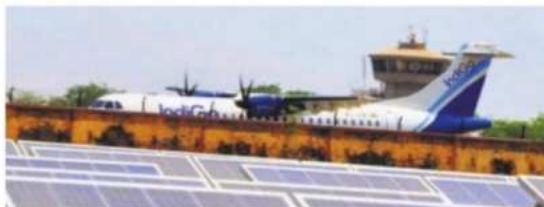
A view of the newly set up solar power plant at Tirupati airport | EXPRESS
