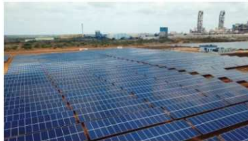
Fourth Partner Energy's 10 MW solar plant at Bharathi Cement's manufacturing facility in Andhra Pradesh
