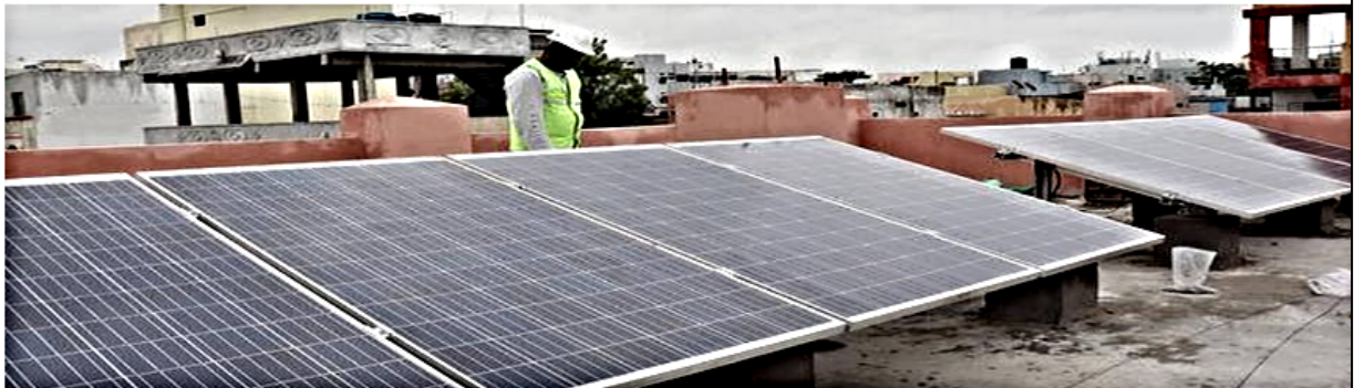
Solar panels set up by 4FPL at Government Primary School, new Bhoiguda, Secunderabad
